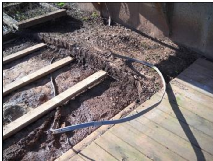
10. Exposed 50amp wire
