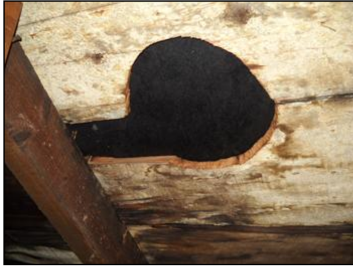
1. Hole in roof planking
